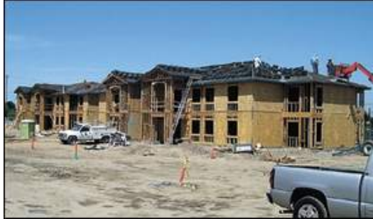
Workers at the Valley Oaks apartment complex walk on top of a two-story building roof. Phase I, which calls for building 81 units, is expected to be completed by December.
